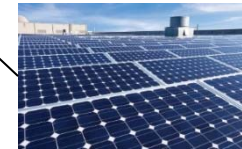
Roof Mount PV
